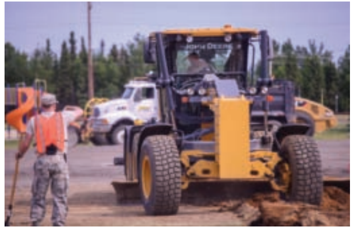
Staff Sgt. Leeman guides heavy equipment, while Tech. Sgt. Brown operates a grader to construct a softball field in Goose Bay, Canada.
