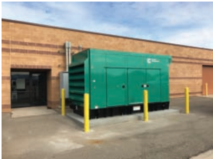
New St. George generator.
