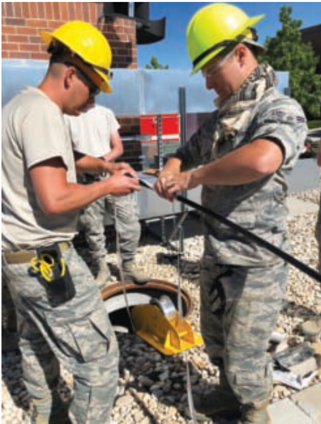
Tech. Sgt. Martin Montano (left) and Airman 1st Class Shane Miller pull fiber-optic cable to support communications and alarms for the munitions storage area at Gowen Field, Idaho.
