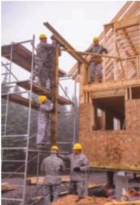
Master Sgt. Moses, 1st Lt. Cross, Staff Sgt. Parkin, Maj. Johnson, Master Sgt. Teuscher, and Capt. Thornton place a load-bearing column for the deck of the cabin in Goose Bay, Canada.
